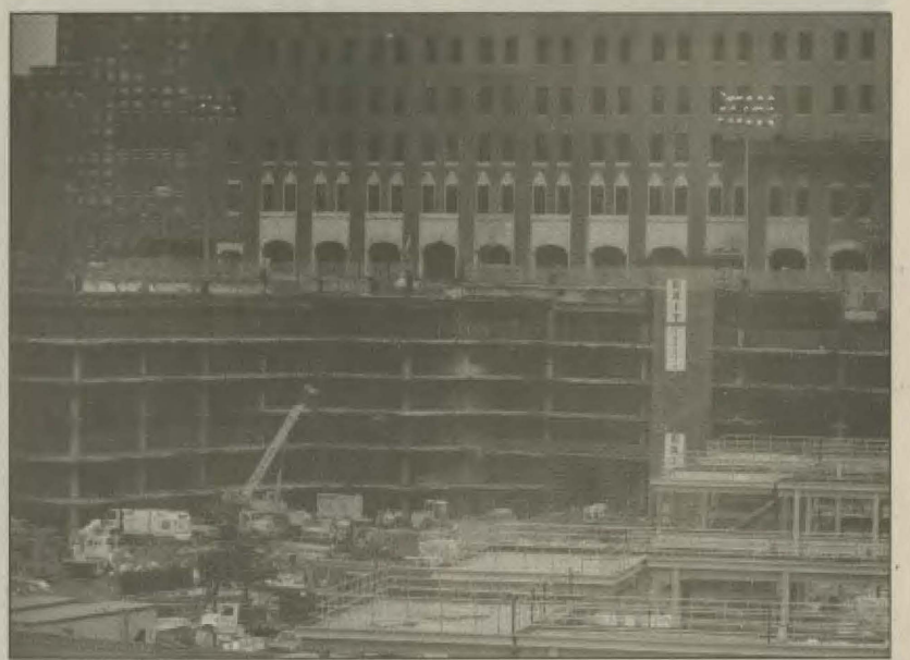
At six stories deep, 'The Pit' is all that remains of the World Trade Center site. Construction vehicles were present in August 2003.
