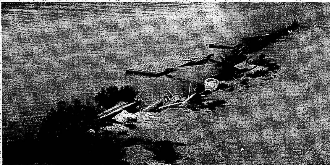
Marist will repair this eroding bulkhead which has already caused deterioration of the area in front of the college boathouse.
