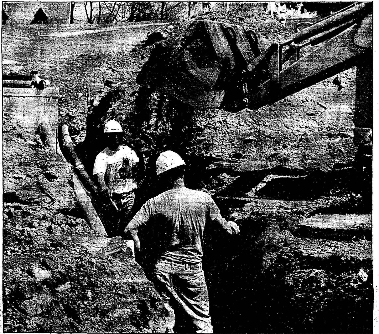
Two construction workers attempt to contain damage done by the fifth water main break this year. See related story.
