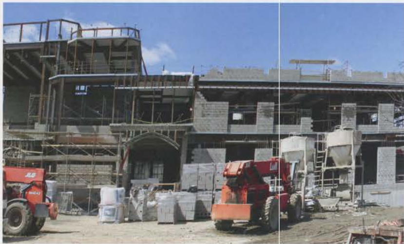
A new academic building is taking shape at the heart of the Marist campus.
