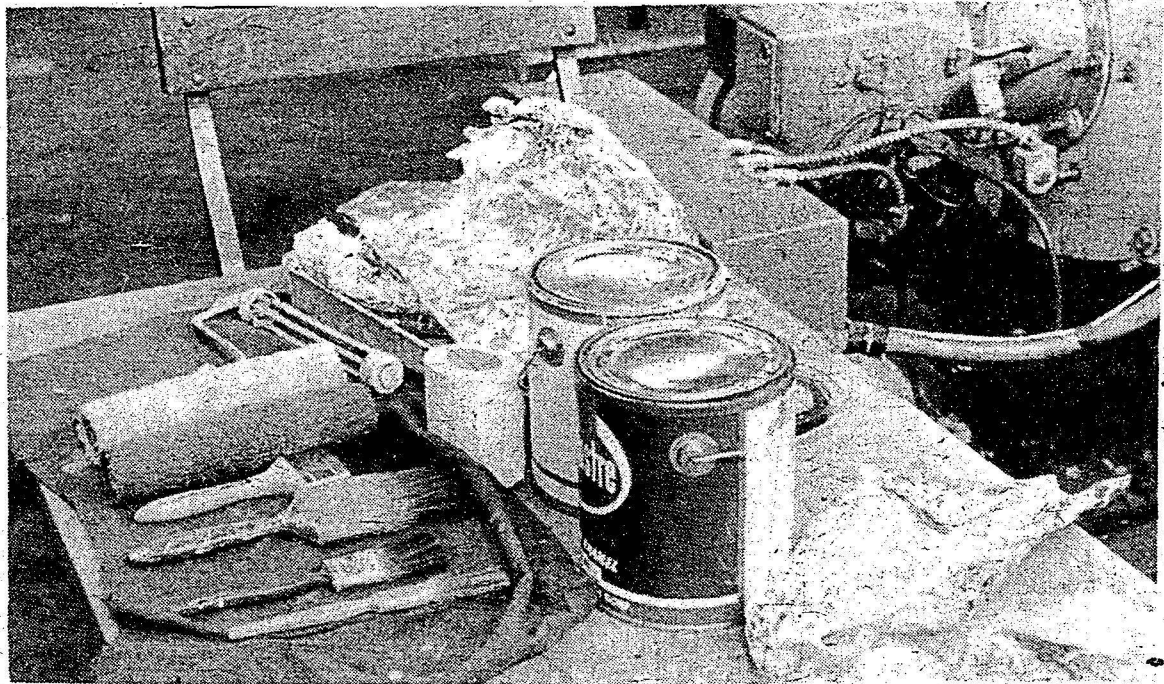
Paint brushes and paint cans in Sheahan Hall boiler room pose a fire threat. photo - Paul Nunziata
