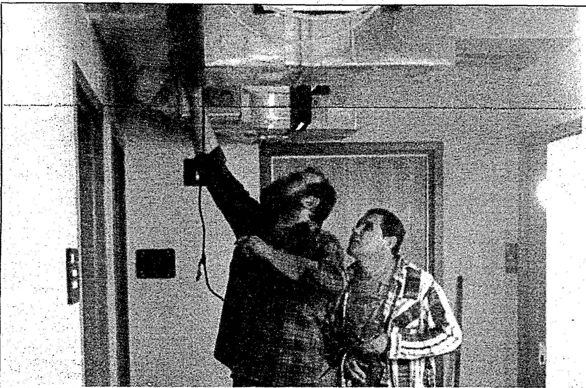
Two unidentified construction workers repair the broken pipe in the basement of the campus center.
