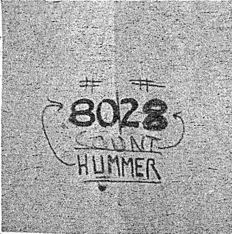
One example of unrepaired damages already paid for by students is this door on the eighth floor Champagnat.
