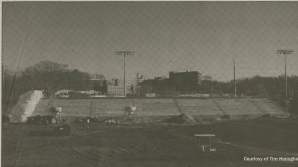
Construction has continued on the new Leonidoff Stadium while all students were home during break. Currently, work has moved along the bleachers on plumbing to get ready to lay down the concrete floor.
